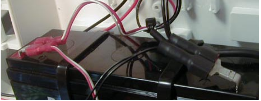
Second Panel power cable connections to the Y-terminal adapters
